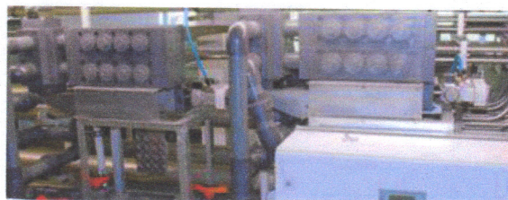
Fig.: 2 pig stations (dark grey boxes), each station controls 4 pigs in 4 different pipelines
